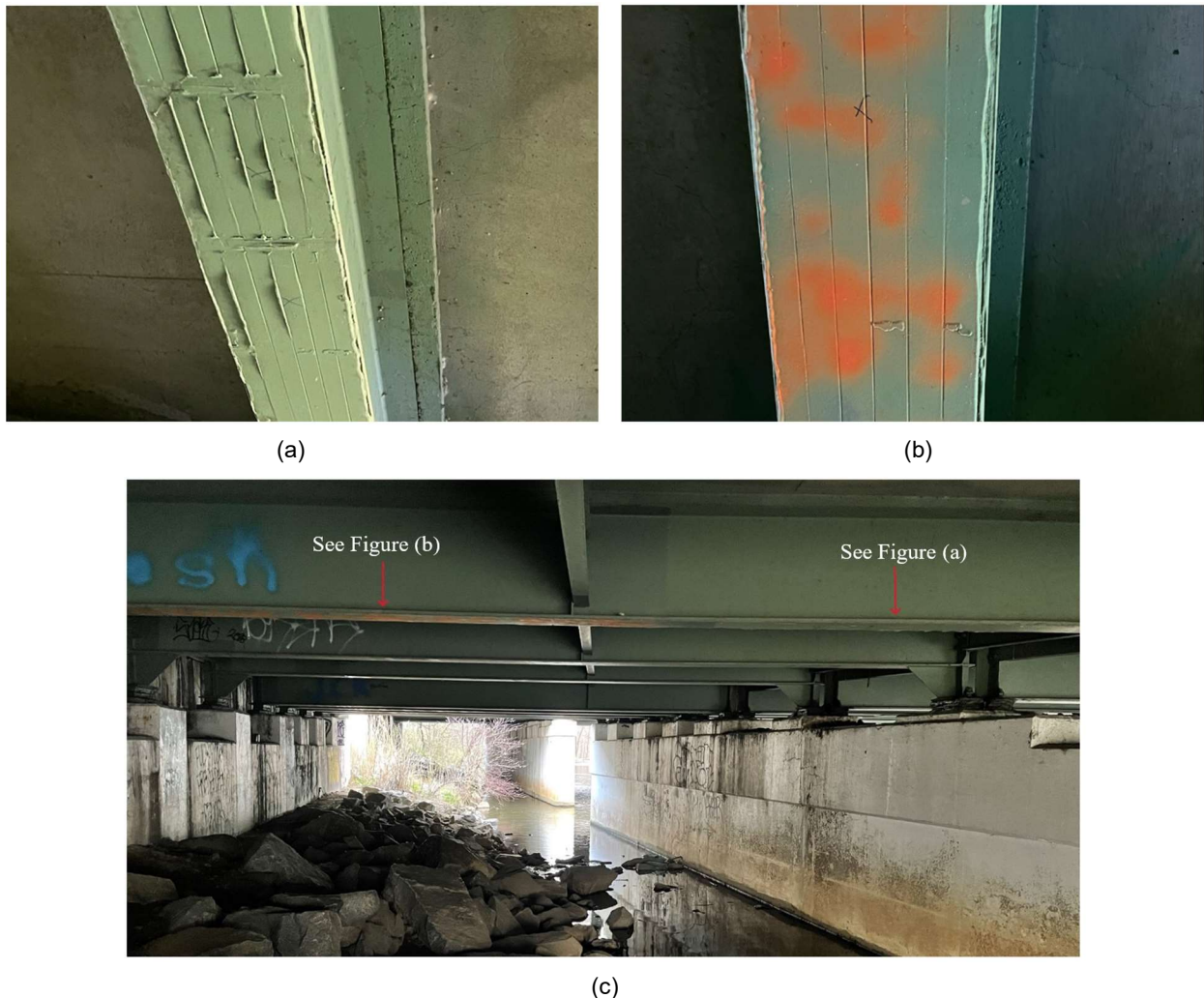
Figure 75. Condition of CFRP composite girder repaired in 2000.
