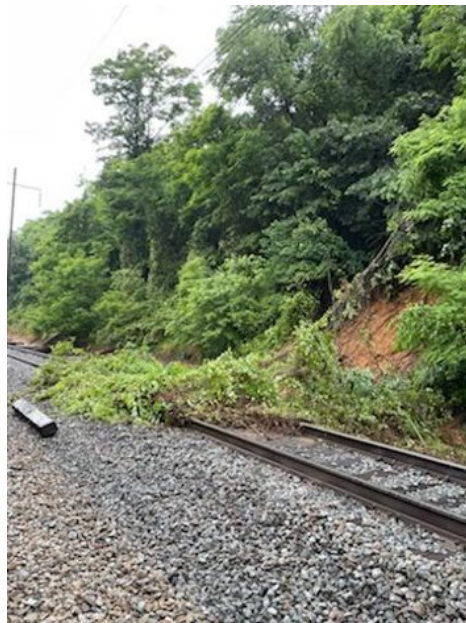
Figure 1.2. A slope failure event near MP 40.5 occurred on 6/8/2021.
