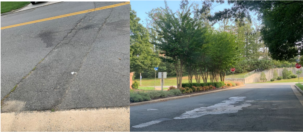
Figure 2. Two Roads with Patching Labels
