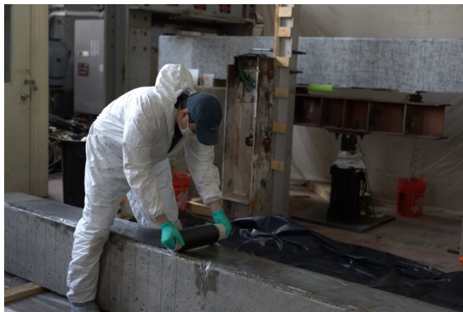
Figure 31. Installing the longitudinal sheet of CFRP onto the tensile face of the girder.
