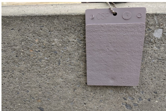
Figure 21. Confirming the CSP of the concrete using an ICRI surface profile coupon.
