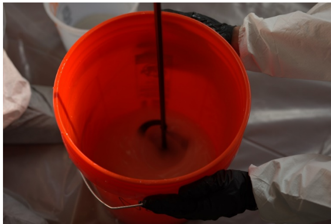
Figure 25. Mixing the epoxy in a 5-gallon bucket using a paddle drill mixer.
