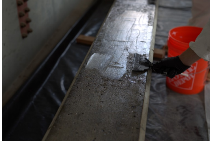
Figure 27. Applying thickened epoxy to the tensile face of the girder using a plastic putty knife.
